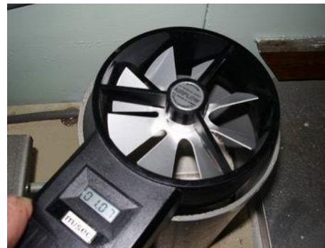
Figure 2: Measuring airspeed through a circular duct
