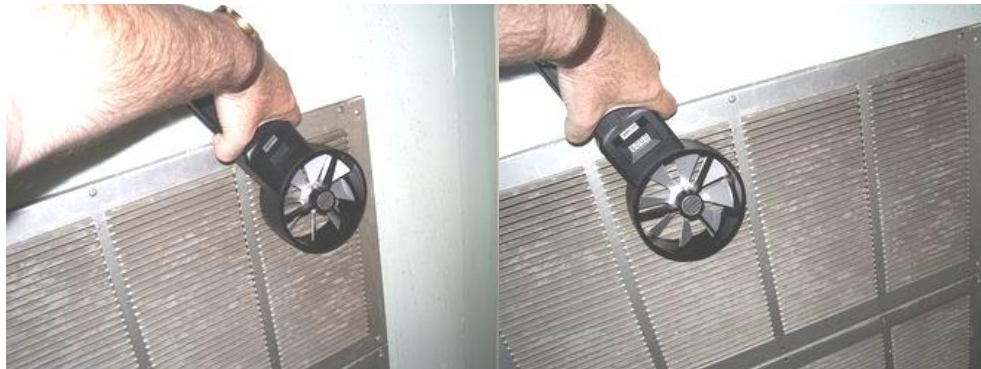
Figure 3: Measuring airspeed through a rectangular vent. Note that for a large vent the average airspeed over the whole vent area must be measured.
